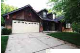
The exterior of a South St. Louis home was in need of roof, siding, and window replacements.
