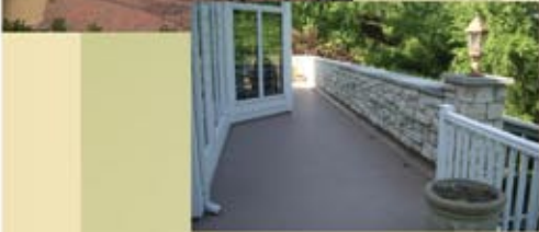
On the deck, the rubber flooring showed signs of water problems.
