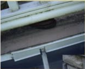
Noticeable cracking in the stone suggested water penetration.
