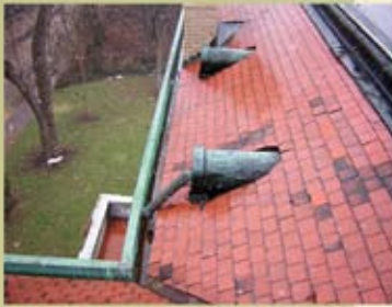
The interior wall leaks were coming from the clay tile roof.
